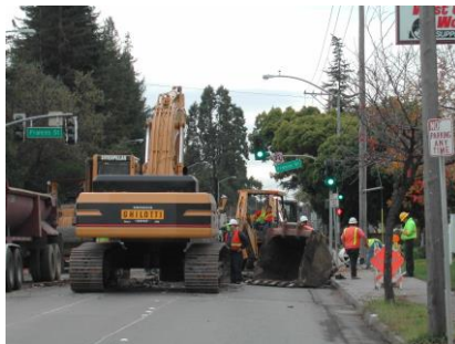
Work Zone Certification Signs & Markings
